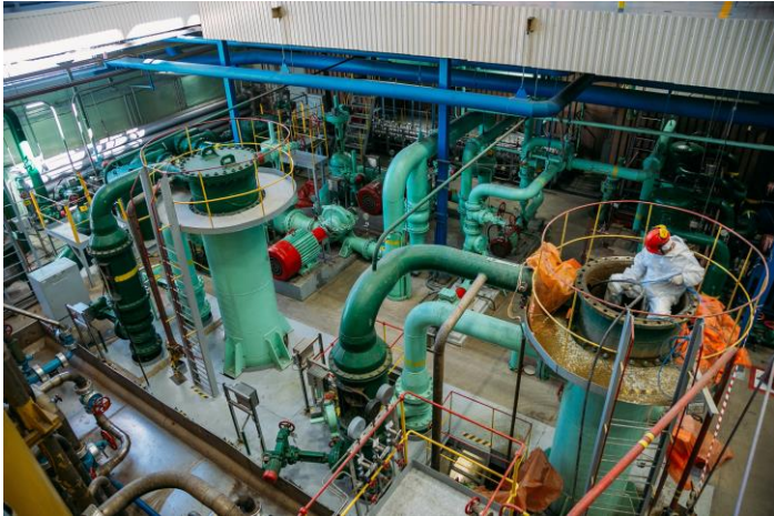
Transport through pipes
