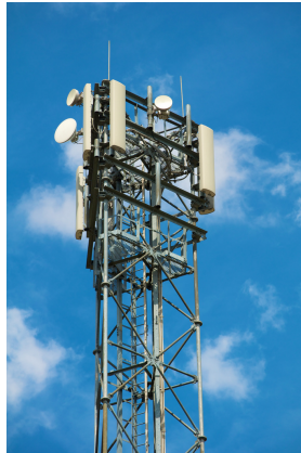
Figure 2.2: Cell tower [Pug10]
