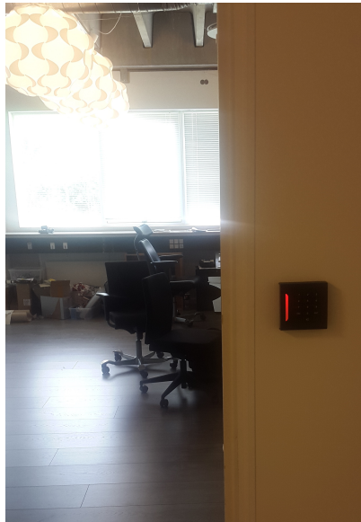
Figure 6.8: Installation of Proximity Reader at one of the AdeoOS Office room
